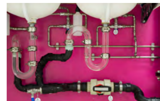
Plumbing facilities providing clear view of blockages in high containment laboratories in the BBSRC National Virology Centre: The Plowright Building. © David Schwalm
